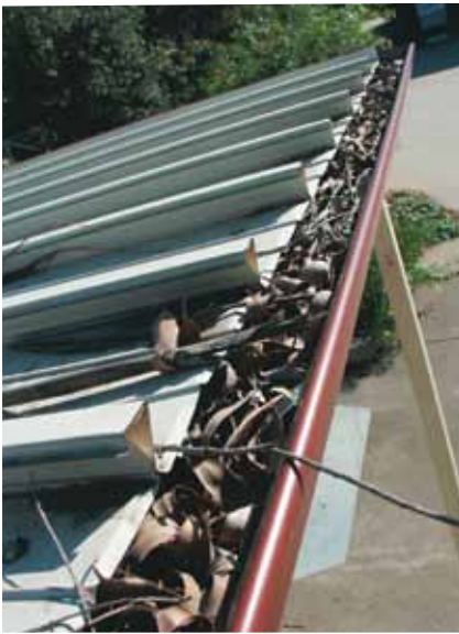
1) A typical suburban gutter clogged with leaf litter prior to cleaning.
