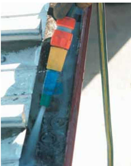
4) Rinse the gutter with water to soften and break up the dirt.
